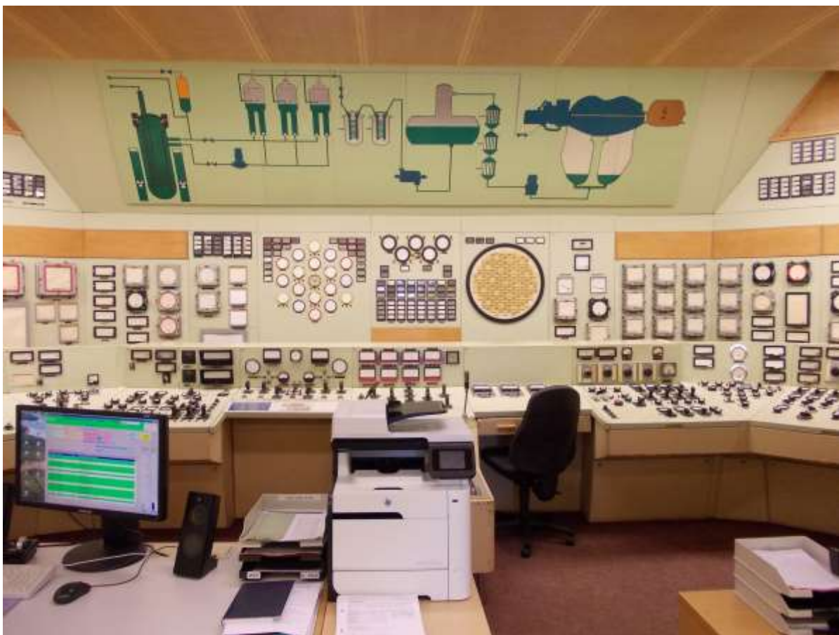
Control room at the decommissioned nuclear power plant in Rheinsberg/Brandenburg
