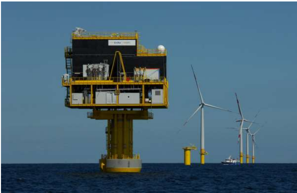
Offshore AC/DC converter platform at Baltic1 offshore wind farm in the Baltic Sea, Germany Photo: 50hertz
