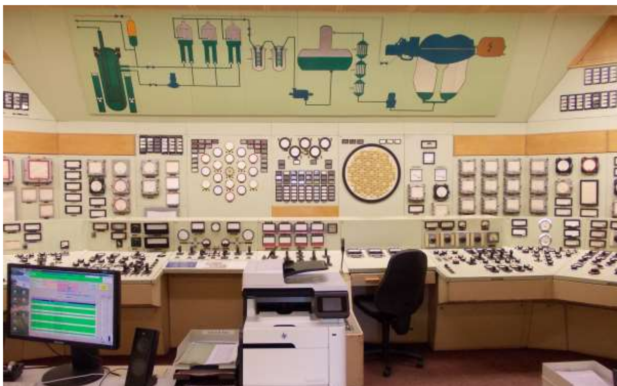
Control room at the former nuclear plant in Rheinsberg
